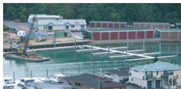
Redevelopment of the western side of Picton's inner marina basin commenced mid-2009 and was completed by year-end; receiving high praise from boaties and locals alike. In addition to replacing the older wooden berths with floating concrete pontoons, the redevelopment included construction of a boardwalk and creation of a public picnic area under the Coathanger Bridge.
